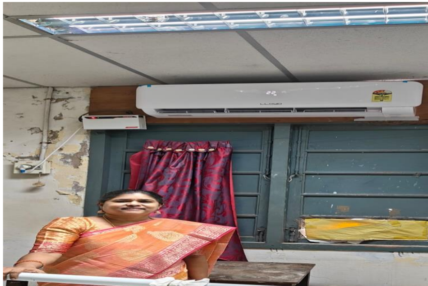
*Air condition one Unit to Pathology Pathology Department
